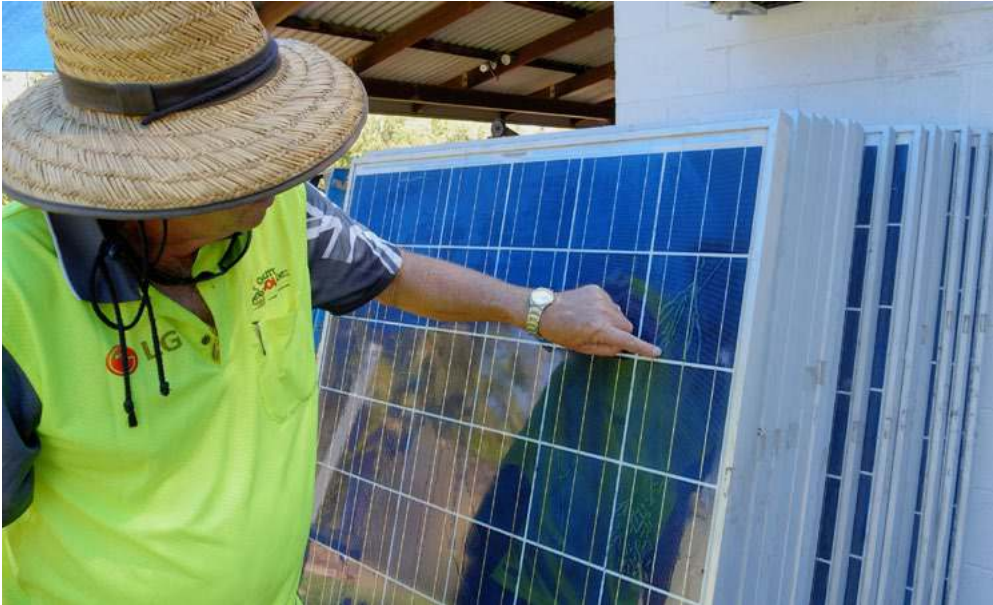
Inspecting cheap panels, that failed after 3 years and were pulled off the roof. The consumer was unable to claim against the manufacturer who had left Australia.
